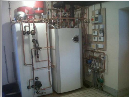
Ground Source Heat Pump
